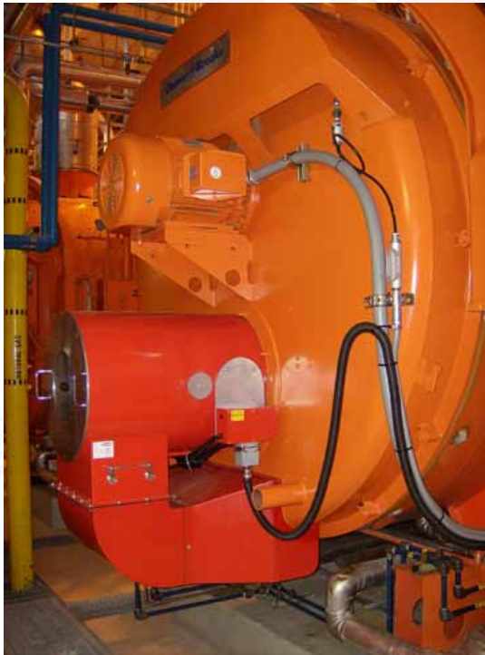
Cleaver Brooks retrofit installation
