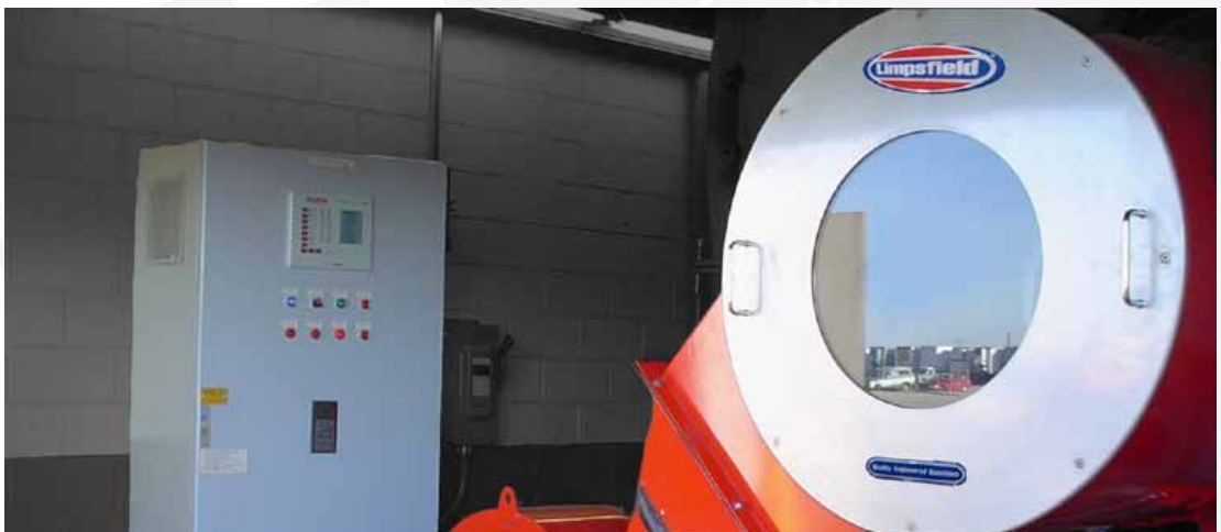
LCN123 Burner on Johnston boiler
