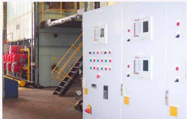
Control panel for a 5 burner application
